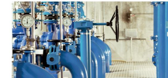
Supplying water for the City of Schwerin
